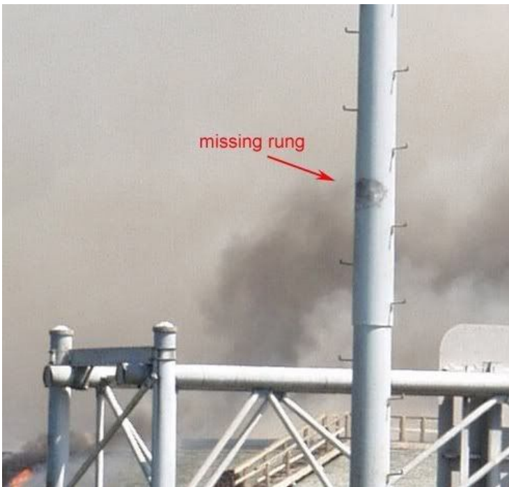
Fig. 2. VDOT camera pole showing damage.
